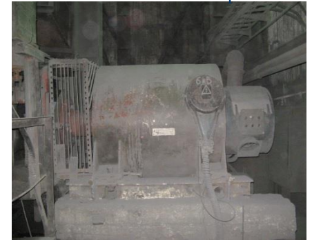
Mill drive at mining and concentration complex
