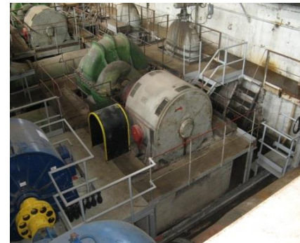
Pump station at heat electric generation plant
